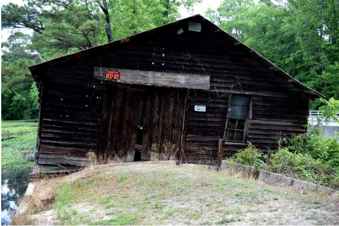
Figure 12. Millhouse addition south elevation showing the concrete retaining wall along the earthen dam/millhouse road; Parker Mill Pond on the left and the NC 96 bridge on the right.
