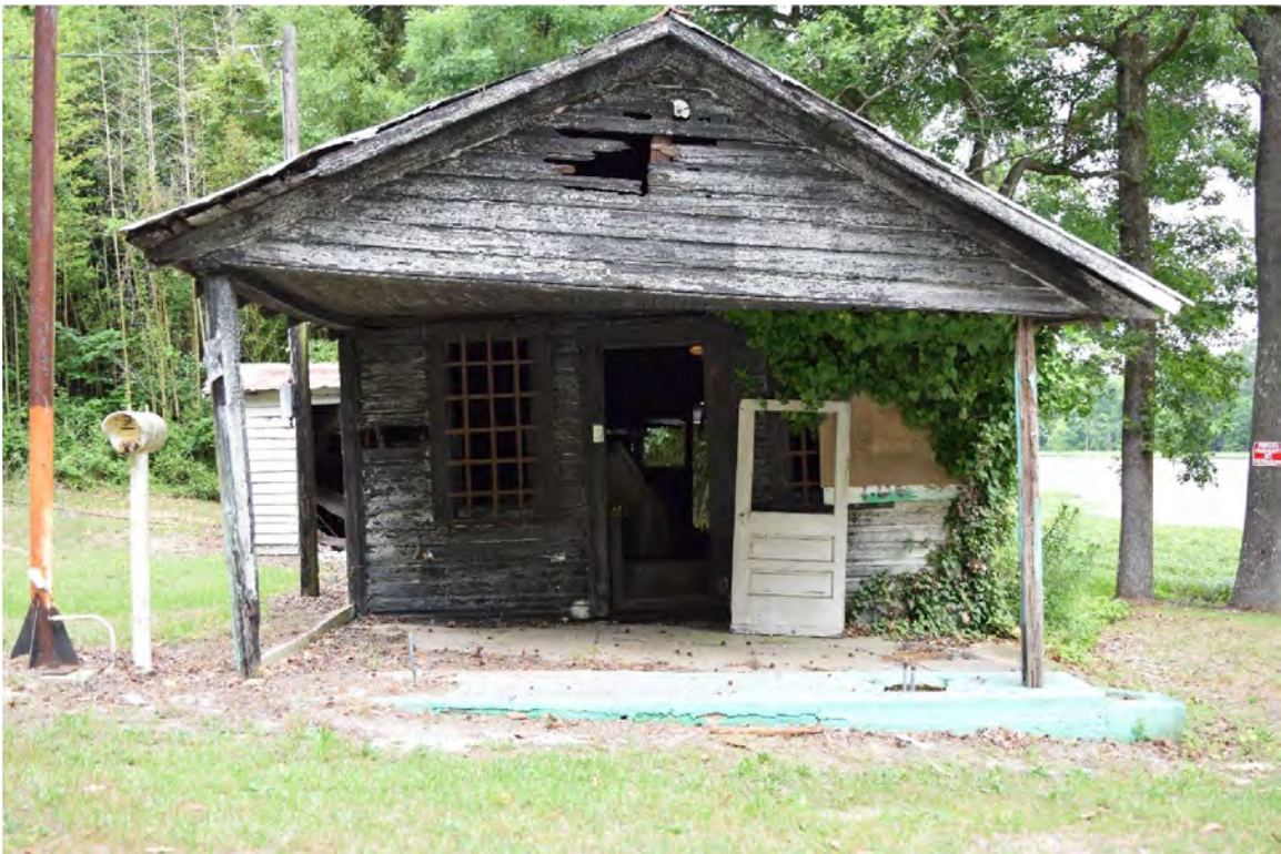
Figure 5. Willie Parker County Store east elevation, Parker Mill Pond in the background.
