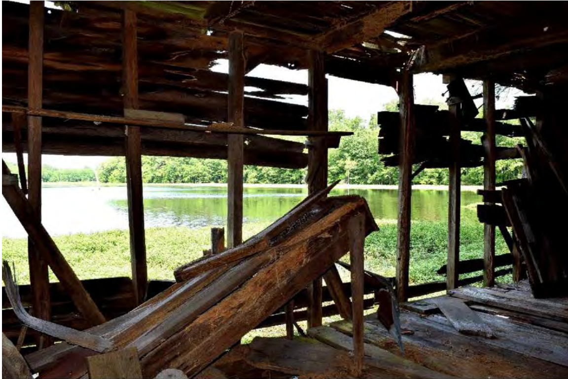
Figure 28. Original millhouse interior, view of the west wall showing the rolling screen. Parker Mill Pond in the background.
