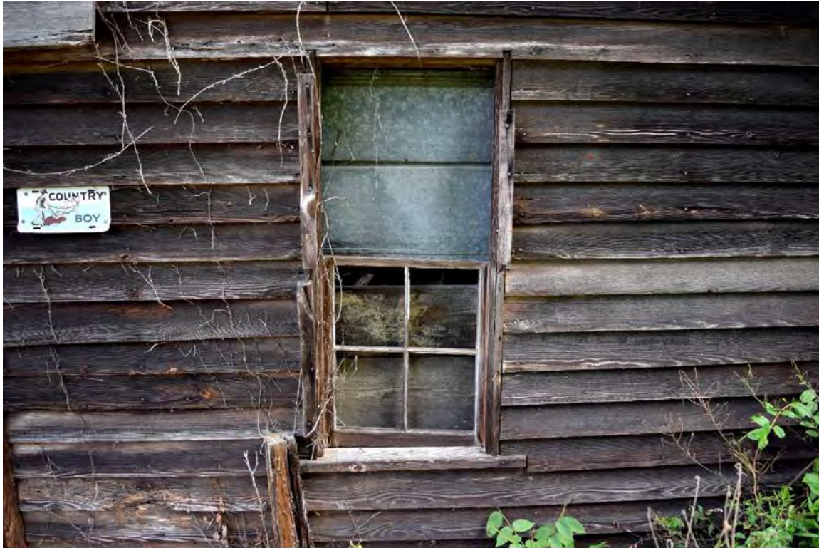
Figure 14. Millhouse addition south elevation, east of the double-door entrance, showing the glazed four-pane sash.
