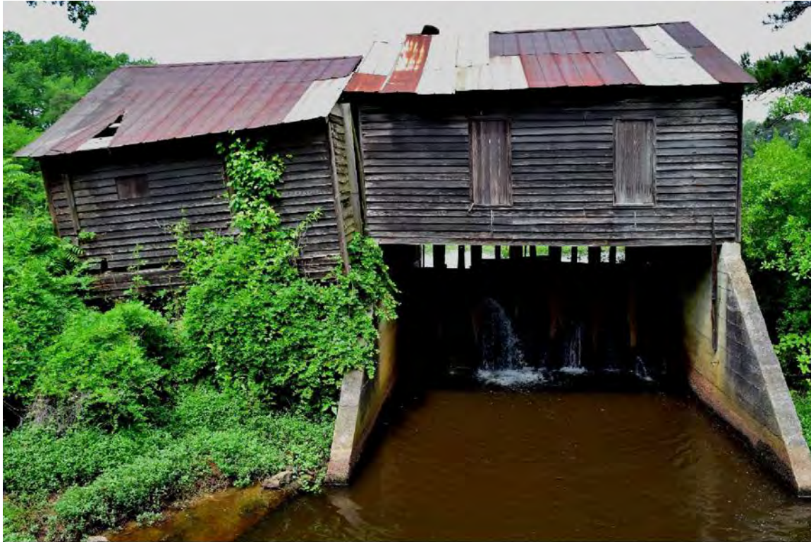
Figure 8. Original millhouse (right) and addition (left) east elevation showing the concrete spillway and wing walls along the tailrace.
