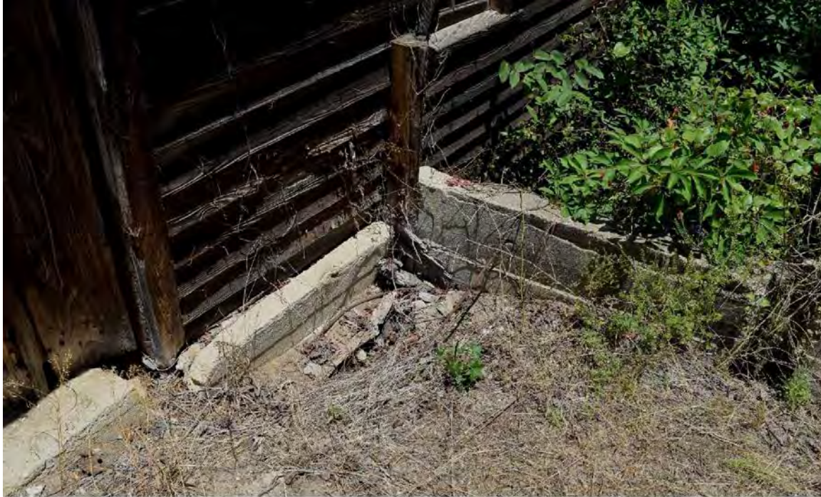
Figure 16. Millhouse addition south elevation foundation detail and concrete retaining wall along the east edge of the millhouse road.
