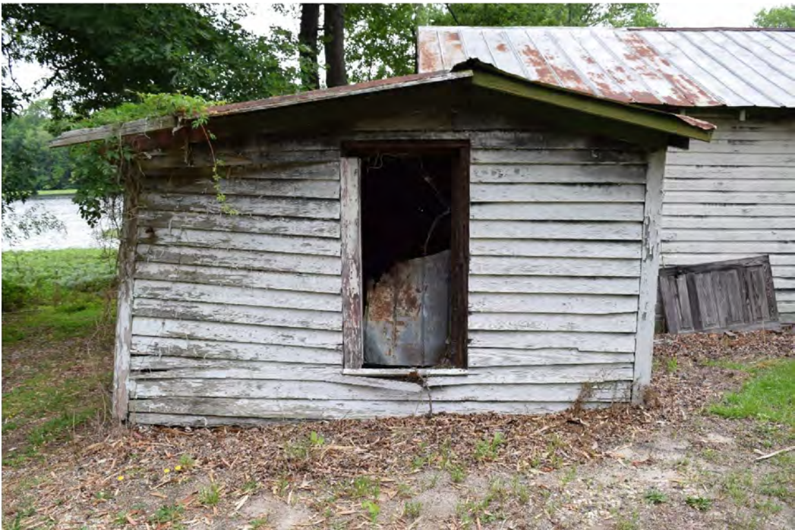
Figure 9. Willie Parker County Store, addition 2 (left) and part of the main structure (right), south elevation.
