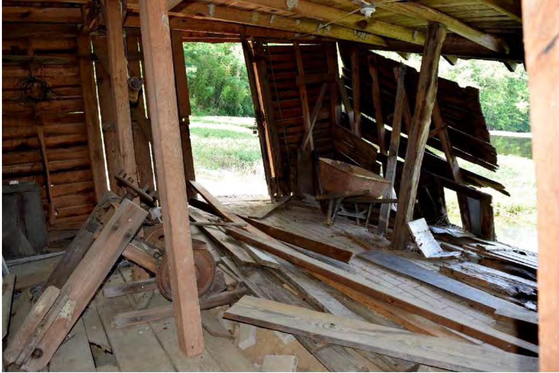
Figure 25. Millhouse addition southwest corner showing the double-door entry and the collapsing west wall.
