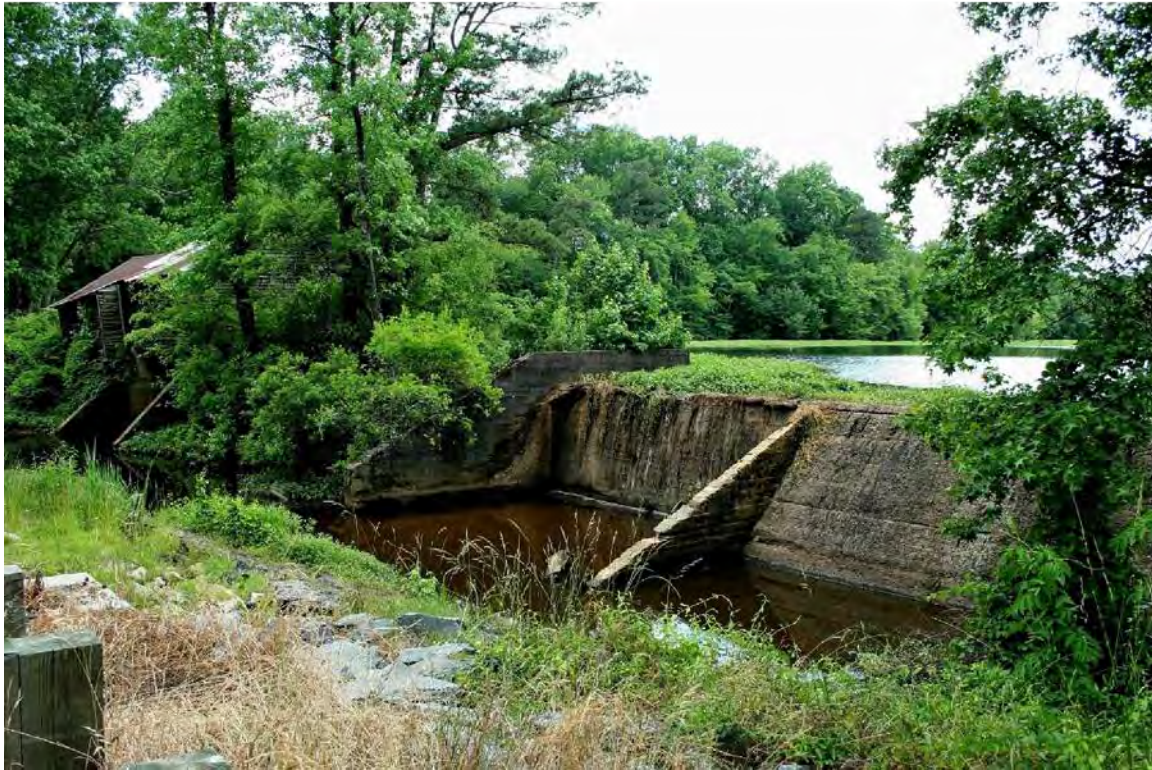
Figure 5. Spillway and millhouse view southwest from the NC 96. Parker Mill Pond in the background.
