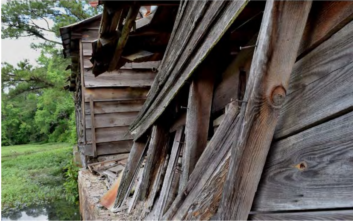
Figure 19. West elevation showing the collapsed addition exterior wall; the original millhouse south elevation is intact and weathered. Parker Mill Pond on the left.
