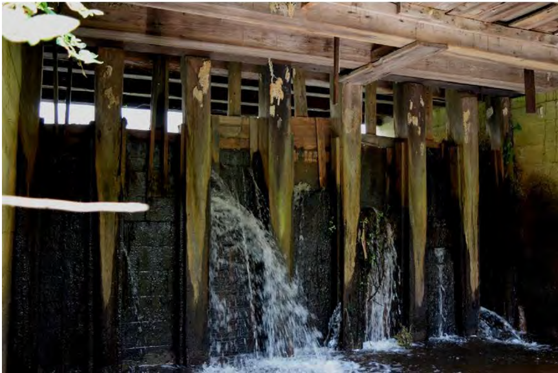
Figure 9. Spillway showing sluice gate below the original millhouse, view from the tailrace.
