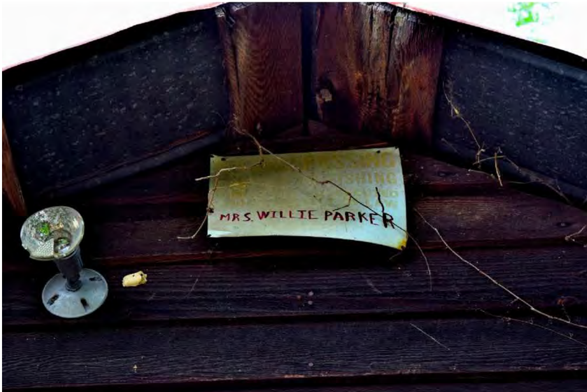
Figure 13. Millhouse addition south elevation showing the “Mrs. Willie Parker” sign at the roof peak.
