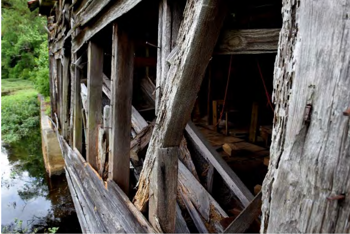
Figure 18. Close-up of the original millhouse west elevation; Parker Mill Pond on the left.
