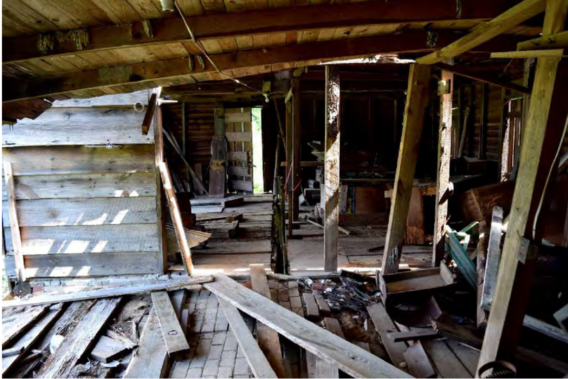
Figure 27. Millhouse interior, view north from the double-door entry on the addition through the original millhouse showing the concrete block floor, the weathered south elevation of the original millhouse building (left) and the opened exterior door on the north wall of the original millhouse.
