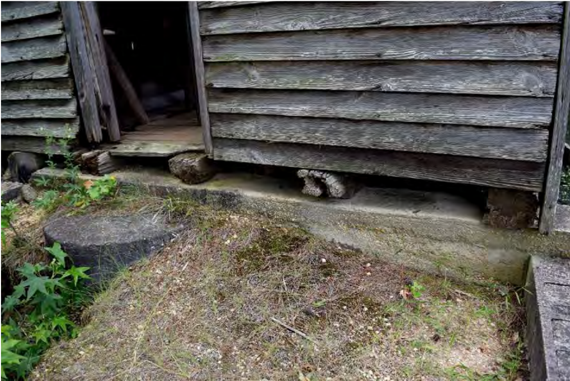
Figure 7. Original millhouse north elevation; foundation detail showing the concrete stepping stone and the cinder block retaining wall along Parker Mill Pond.
